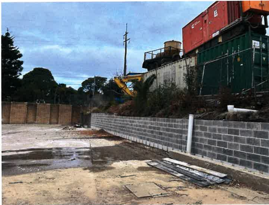
Figure 3 – Water overflow onto 109 assumed to be from 109A at present
